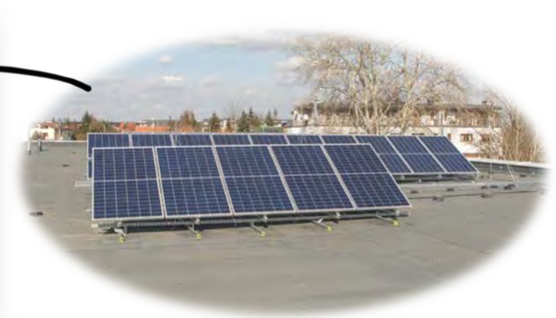
Photovoltaic installation power 9,6 kW
